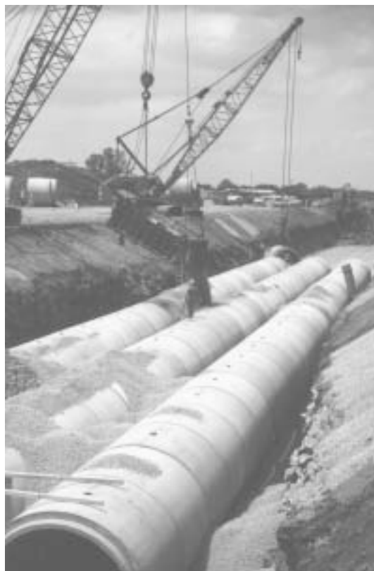
A dump truck bed equipped with an air-controlled gate was used to accurately place the bedding material, #57 crushed stone.
