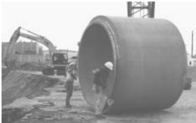
New joint ring forms allowed as many as 24 pieces of 108" pipe to be manufactured per day using only 12 sets of rings.
